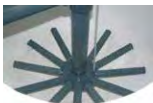
Collector arms detail
