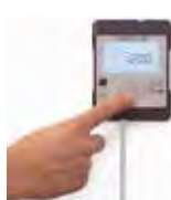
HMI control system on wall
