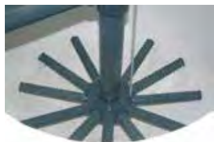
Collector arms detail
