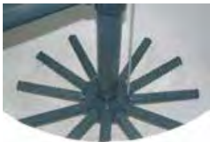
Collector arms detail
