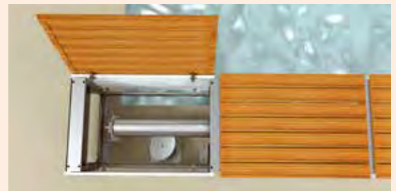
Access to the skimmers and mechanical parts
